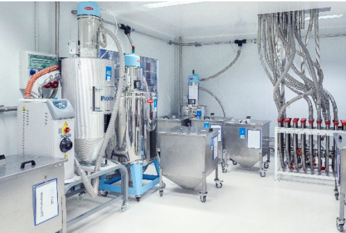
Raw material distribution room
